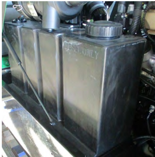
Figure 10.1-1 Fuel tank for Diesel engine
