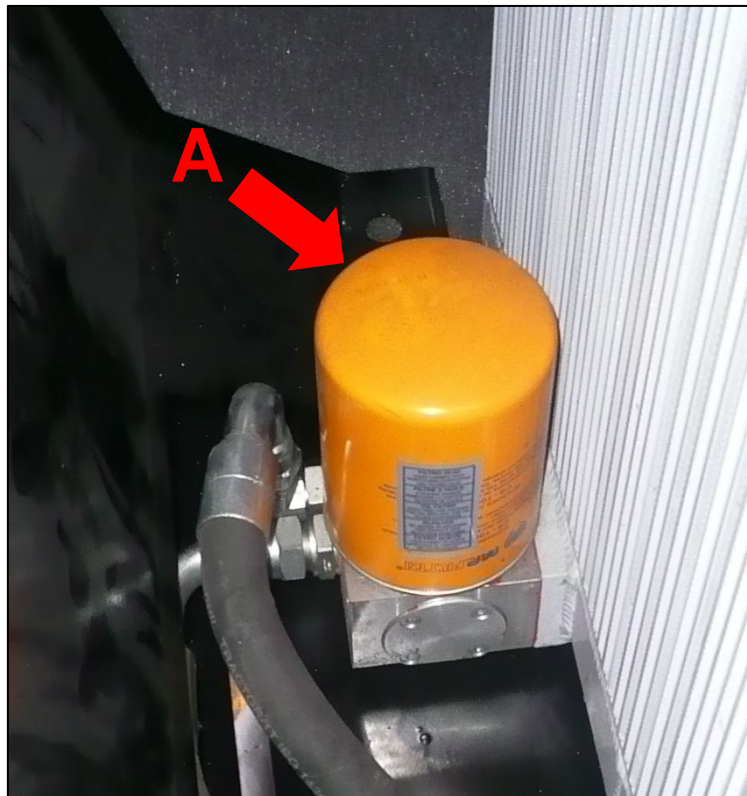
Figure 13.4-6 Compressor oil filter
