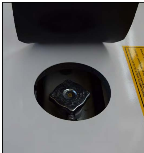
Figure 10.1-3 Checking the radiator antifreeze
