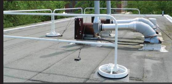
HVAC / ROOFTOP EQUIPMENT
