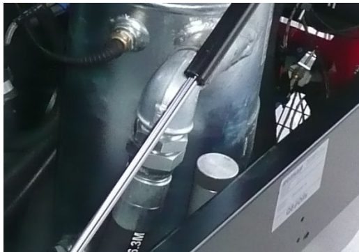
Figure 10.1-1 Checking the oil level in the compressor
