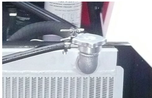
Figure 10.1-3 Checking the radiator cooling liquid
