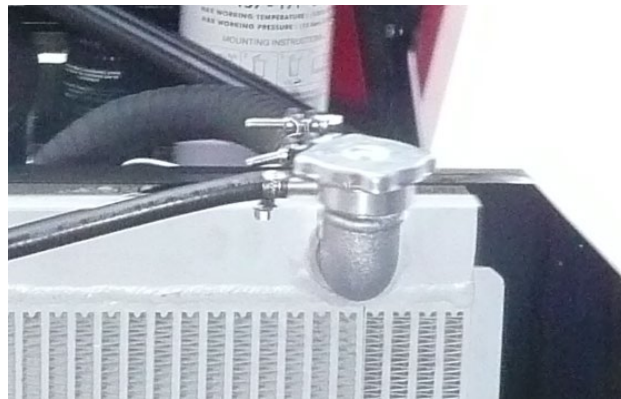
Figure 13.4-3 Checking the coolant radiator
