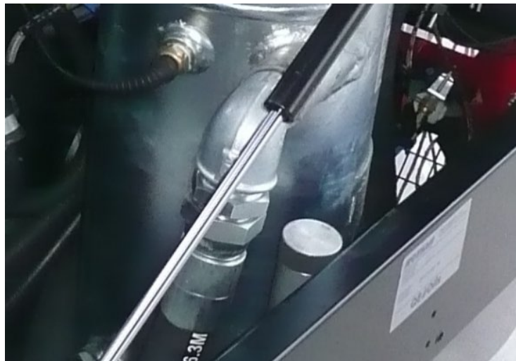
Figure 10.1-1 Checking the oil level in the compressor
