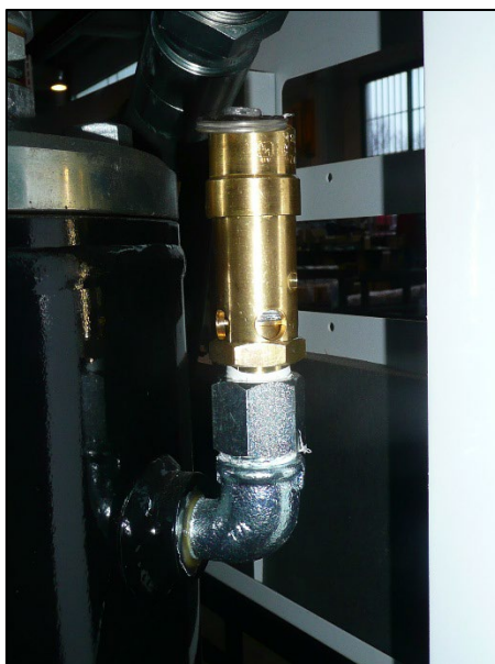
Figure 12.1-1 Control of the safety valve
