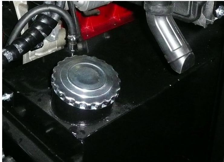
Figure 10.1-2 Gas oil tank for Diesel engine
