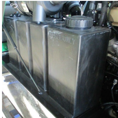
Figure 10.1-2 Fuel tank for Diesel engine
