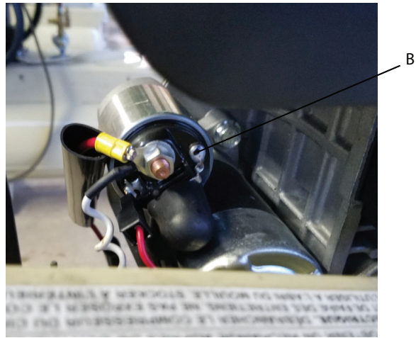
Yanmar Diesel Engine Battery (+) Positive cable connection point.
