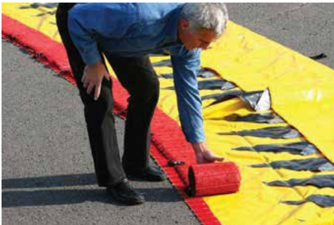
3 - Place a second series of ballast weights along the entire length to prevent water infiltrations.
