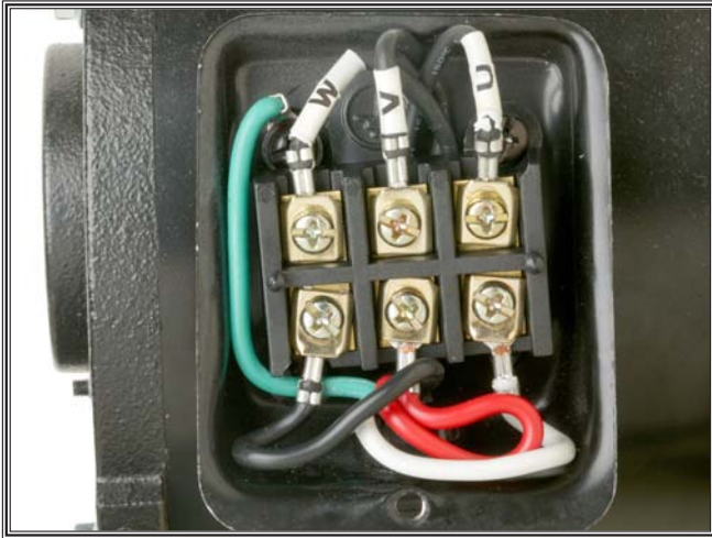
Figure 58. Motor junction box wiring.
