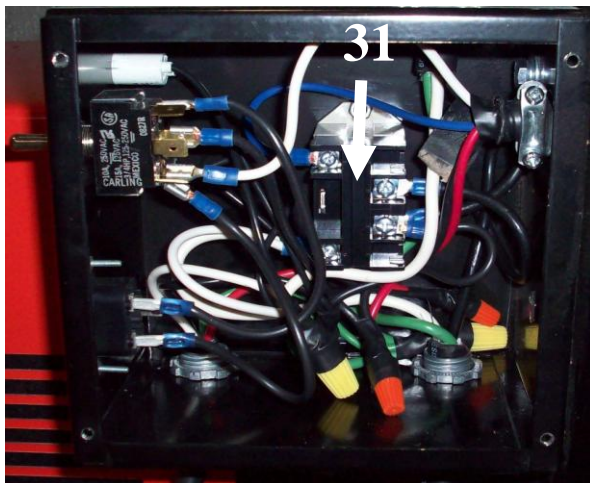
Inside Control Box
