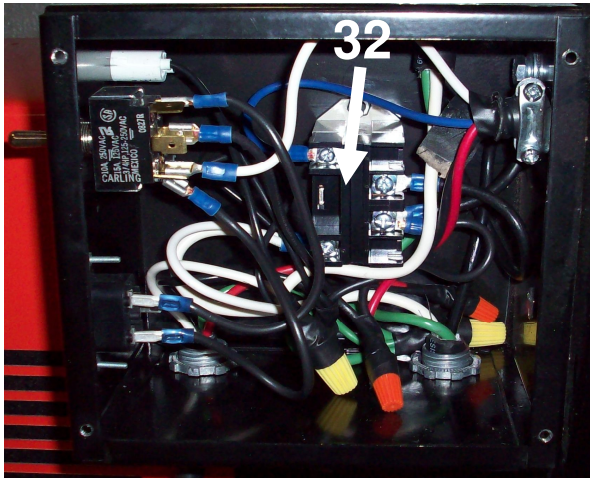
Inside Control Box
